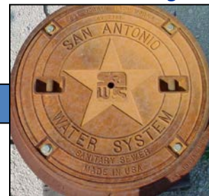
Sewage Collection System
